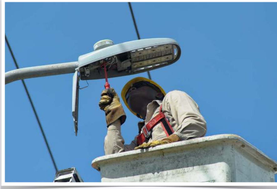
JPS Lineman works on LED streetlight on Brunswick Ave in Spanish Town
