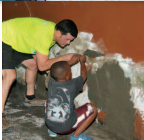
Cadell gets the hang of the preparing the wall for rendering with President & CEO, Mr. Emanuel DaRosa (left).
