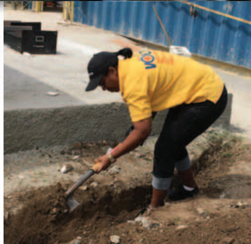
Customer Care Manager at the Spanish Town Customer Service Office, Debronnette Dixon, got busy on Labour Day, as the team worked on a ramp for the Portmore Self-Help Disabilities Organization.
